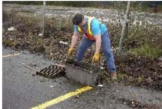
Figure 6.16-7. Maintenance of a bag type water quality insert, (Full Circle Ag, Inc., http://www.fullcircleag.com/pages/954364/ ).
