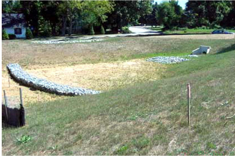
Figure 6.15-2 Picture of a sediment forebay created with a riprap berm. Although not shown, it is recommended that sediment forebays be vegetated with a minimum of native wet meadow planting, however more substantial plantings are preferred. (Chester County Conservation District photo, 2002)
